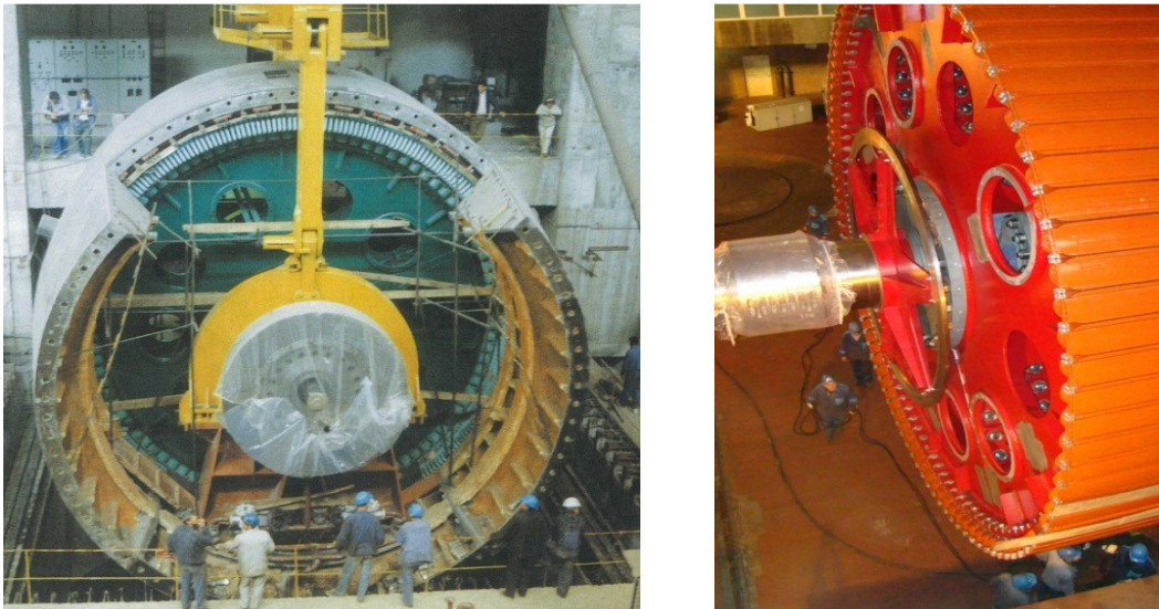
Fig. 5. Generator stator and rotor
