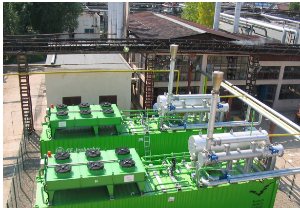
Fig. 1. General view of the cogeneration plant
