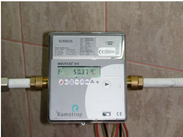
Figure 5 – The energy meter
