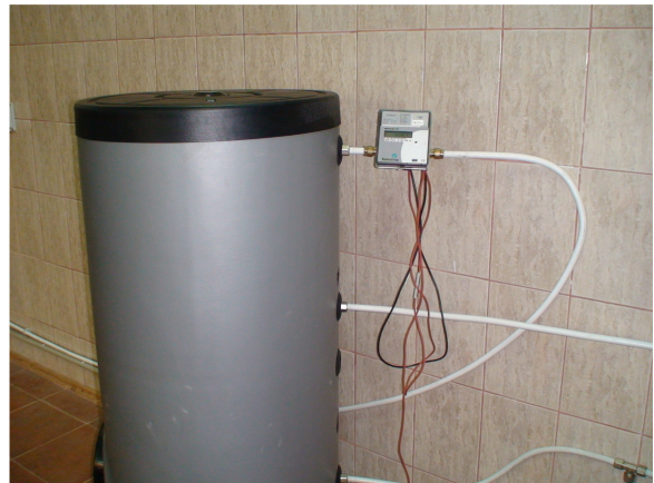
Figure 6 - The solar boiler
