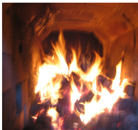
Fig. 4. The flame in the 80 kW boiler furnace
