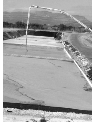
Fig 6 Dry ash and sludge landfill
