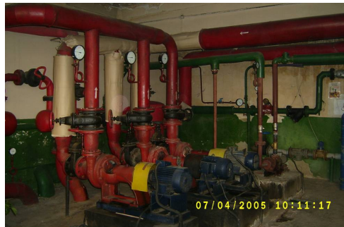
Figure 3 Old district heating thermal sub-station in Iasi [3]
