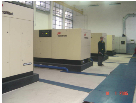
Figure 2 New compressed air station [3]
