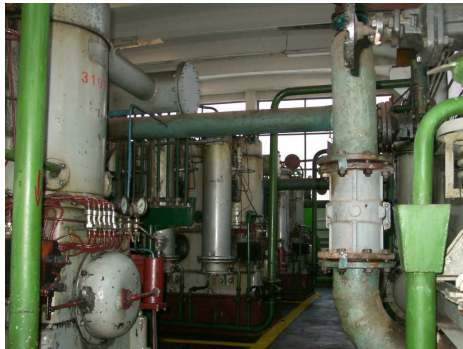
Figure 1 Old compressed air station [3]
