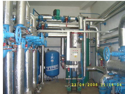
Figure 4 New district heating thermal sub-station in Iasi [3]
