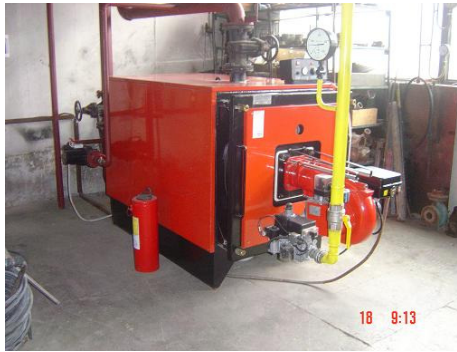
Figure 10 The heating plant installed in Arc Dorohoi [3]
