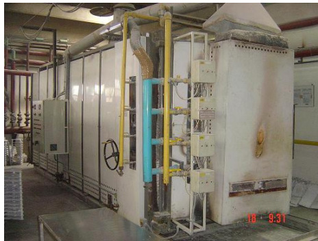
Figure 9 The glass furnace installed in Arc Dorohoi [3]
