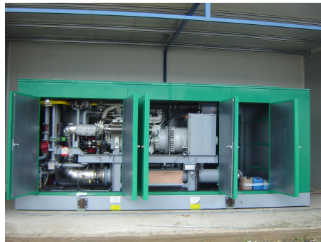
Figure 7 The co-generation unit installed in CarmOlimp Ucea de Jos [3]
