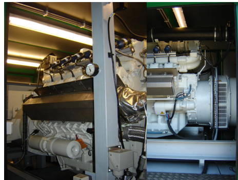
Figure 8 The co-generation unit: engine type MAN E 2842 LE312 [3]
