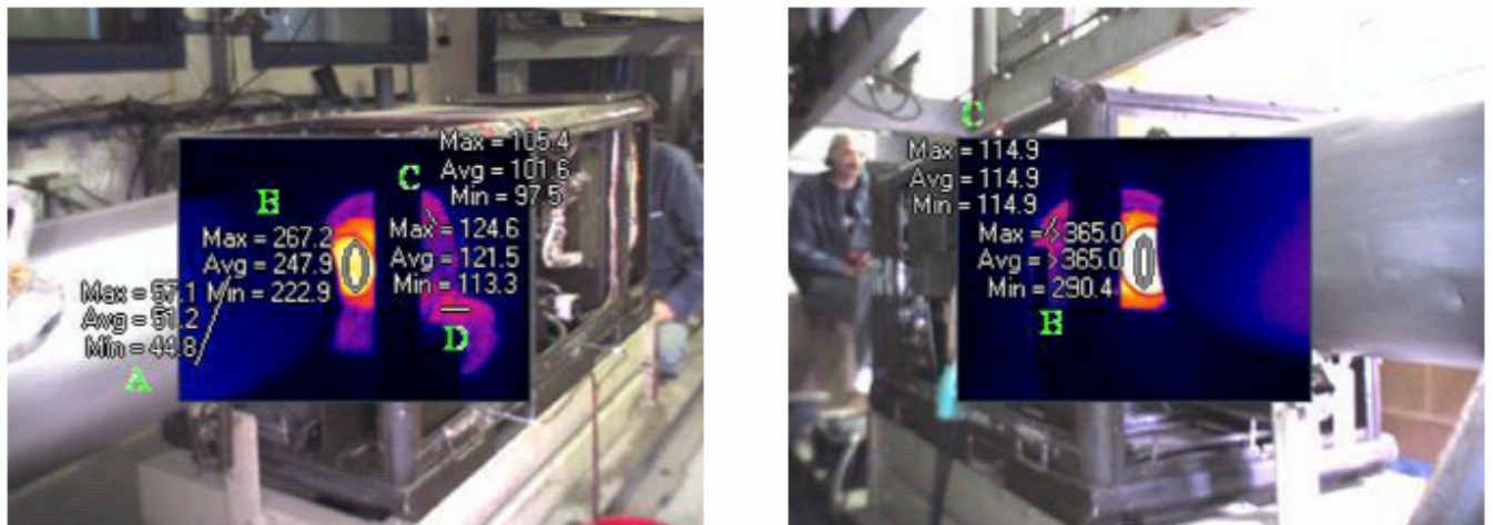
Figure 8: Electrical generator temperature
