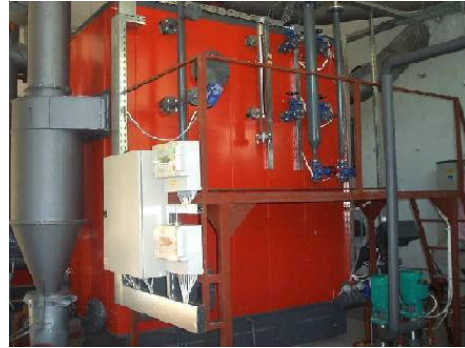
Figure 6 New wooden pellets fired BINDER type boiler
