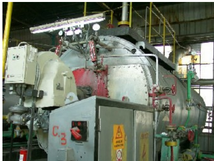
Figure 3 Natural gas fired old steam boiler
