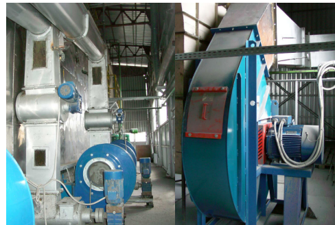
Figure 4 Sunflower peels fired new steam boiler
