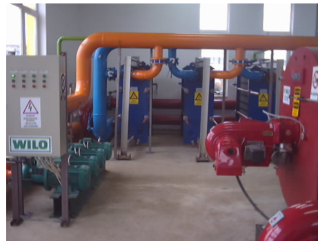
Figure 2 Geothermal station after modernization [3]
