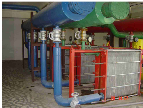
Figure 1 Geothermal station before modernization [3]
